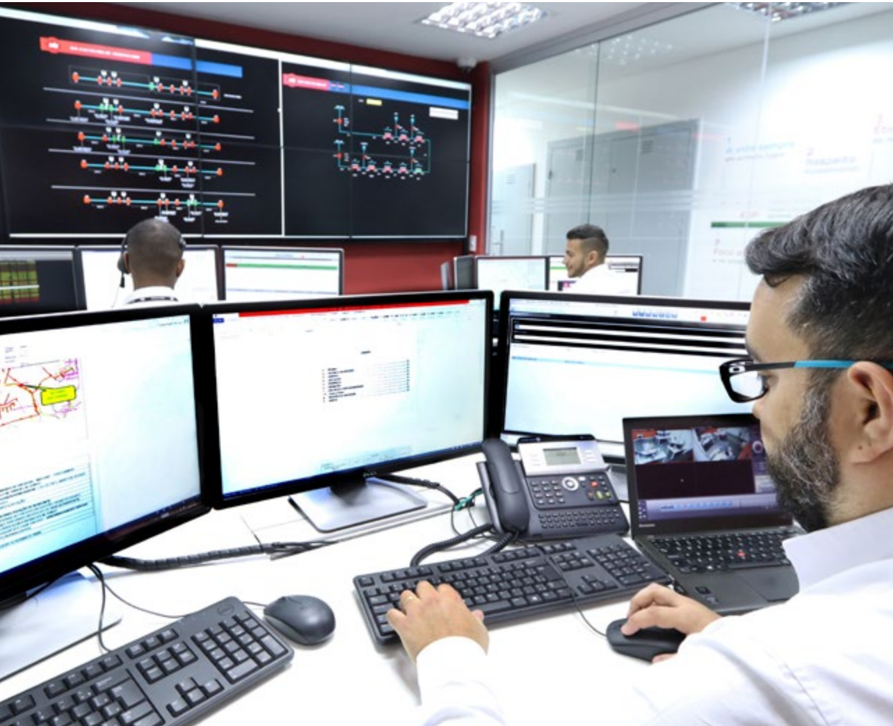
EDP São Paulo operational control
