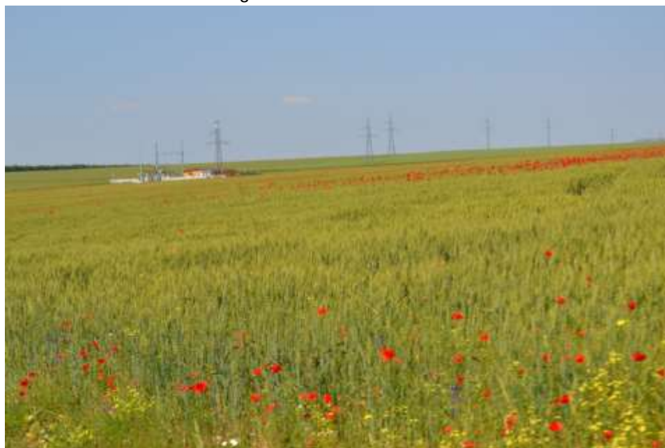
Fig. 8 – statia electrica Sarichioi
